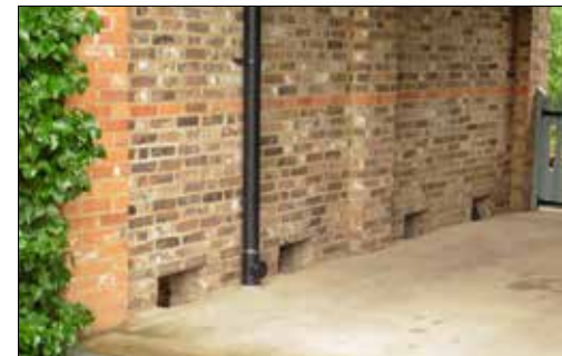
Example of openings in a boundary wall to allow water to pass through it in the event of flooding, and decorative brick banding
