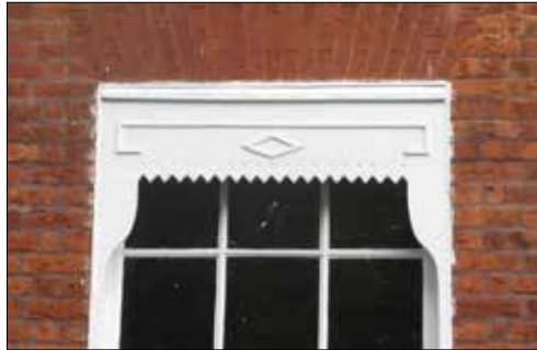
Example of blind boxes (originally containing larger sun shades) on a period property in Datchet
